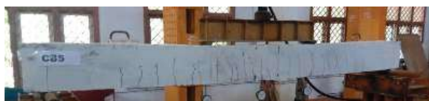
Fig.7. Crack Pattern of Beam
