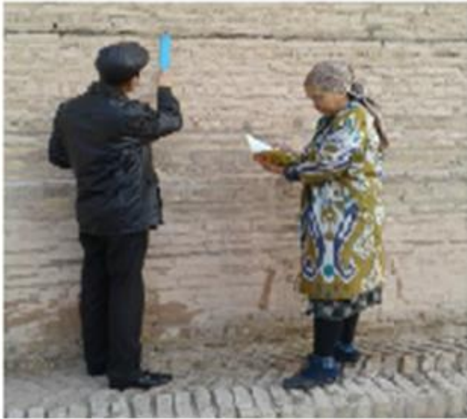
Figure 5. Observation of termite damage to the cane covering between the main wall and the foundation on the south side of the Matpanaboy madrasa (November 2017).
