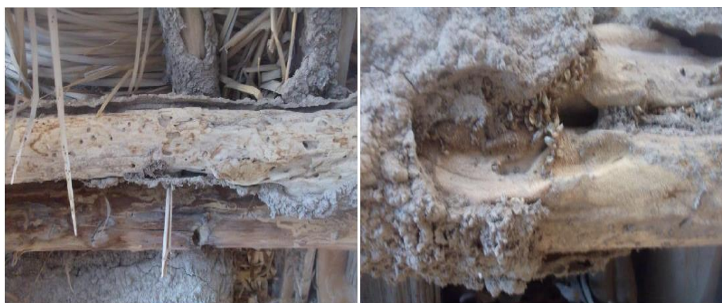
Figure 7. Building materials found to be damaged by termites.
