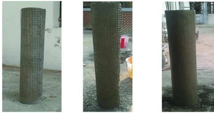
(a) Wrapping the Column with Square Wire (b) Application of Flowable Mortar (c) Ferrocement jacketed column
